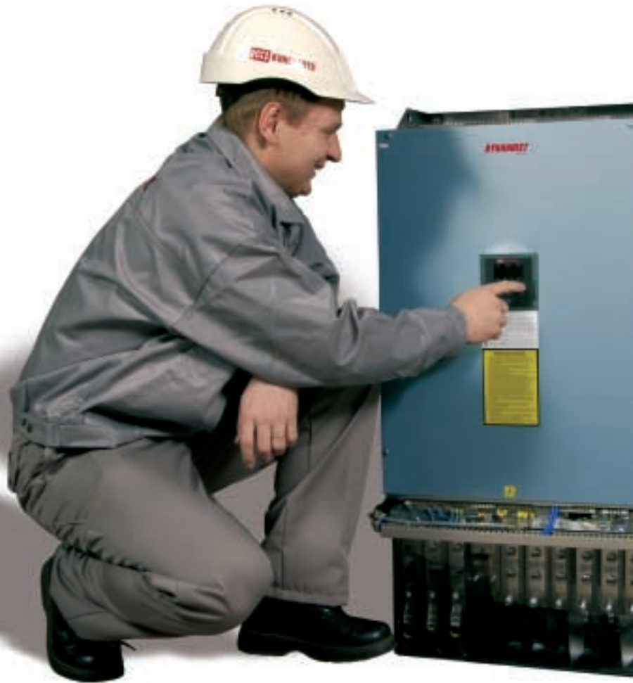
KCI Konecranes' harbour crane maintenance business, KCI Koneports, is rapidly increasing in importance for new crane sales. In the picture, Jukka Tukia, Service Engineer, inspects the electric panels in a RTG controls room.
