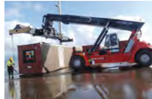
REACH STACKER LIFTING CONTAINER HOUSE MODULES using slings attached to the standard lifting eyes.
